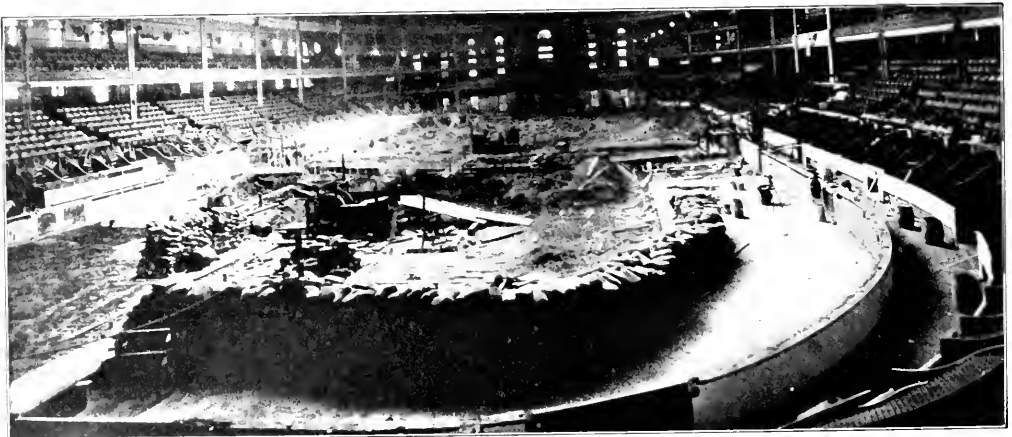
FIG. 28. ON MAY 28 THE RETAINING WALL HAD BEEN POURED AND STRIPPED OF THE FORMS; BULKHEAD DOORS HAD BEEN PUT IN PLACE. TILE WAS BEING SET ON THE RETAINING WALL. MARBLEOID FLOORING FOR THE PROMENADE DECK HAD BEEN COMPLETED. FLOOR SLAB OF MASS CONCRETE WAS BEING POURED. ON THE EXTREME LEFT THE MEMBRANE WATERPROOFING WAS BEING APPLIED TO THE SLAB. THE FORMS IN THE DEEP DIVING POOL WERE IN PLACE AND HAD BEEN POURED. THE ENTIRE ARENA FROM CEILING DOWN, INCLUDING ALL CHAIRS AND SEATS, HAD BEEN PAINTED
